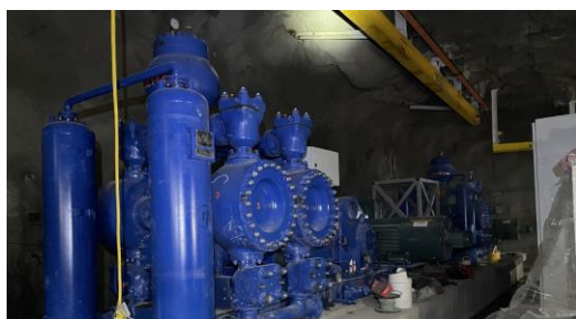
Geho Pumps installed and mechanically complete
